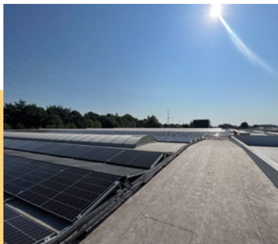
Ets Joskin equipped with an integrated energy system including 3,800 photovoltaic panels, 3 storage batteries and 26 recharging points for electric vehicles.
