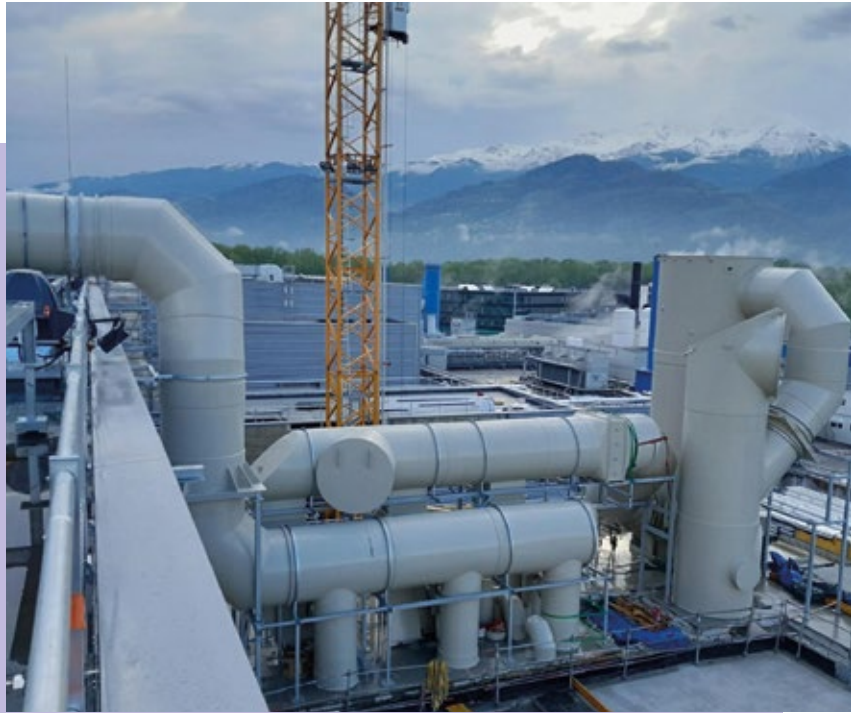
John Cockerill supplied gas scrubbers to treat discharges from a new French plant of a semiconductor manufacturer.
