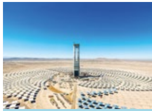
Solar Tower Receivers & Steam Generators
