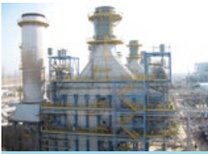
Heat Recovery Steam Generators
