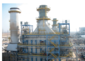
Heat Recovery Steam Generators
