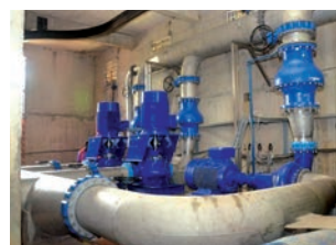
Station de pompage d'eau potable, 850 m 3 /h (Ndogbong, Cameroun)
