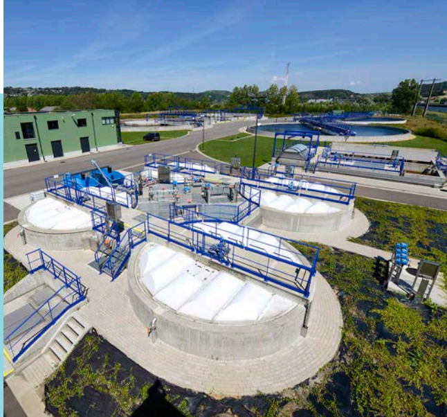
Municipal wastewater treatment plant, 54 000 PE (Amay, Belgium)
