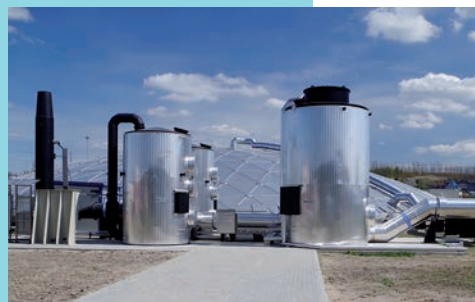
Odour treatment in wastewater treatment plant (insulated installation), 48 000 m 3 /h (Poland)
