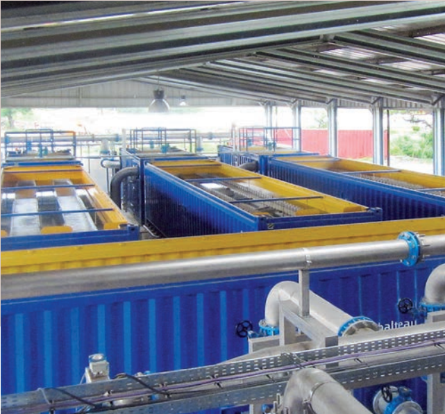
Drinking water treatment plant, containerized units, 750 m 3 /h (Kpong, Ghana)
