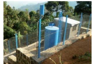
Drinking water treatment plant, fully hydraulic driven 20 m 3 /h (Jikejemoku, Cameroon)
