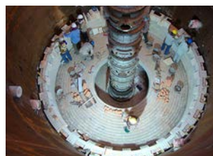
Multiple hearth furnace (MHF), The Nesa Solution®
