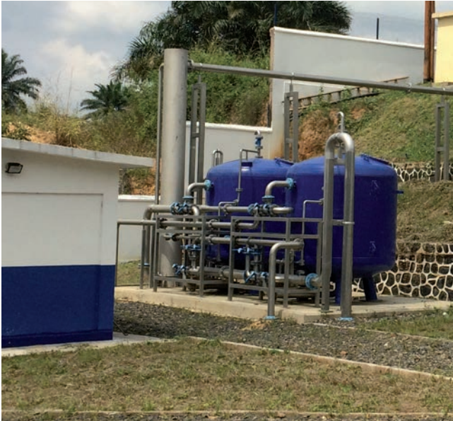
Drinking water treatment plant, 50 m 3 /h (Tonga, Cameroon)
