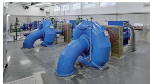
Hydropower plant, 2.3 MWatt (Eupen, Belgium)
