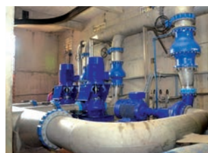
Drinking water pumping station, 850 m 3 /h (Ndogbong, Cameroon)
