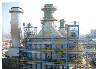
Heat Recovery Steam Generators
