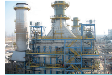
Heat Recovery Steam Generators
